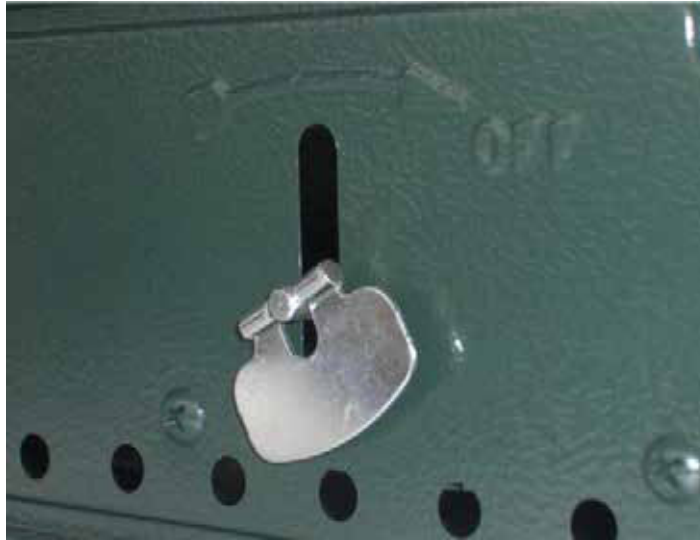
Figure 8 Auxiliary Burner Control
